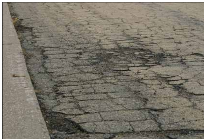
Figure 5. Some of Cuba City's road require maintenance
